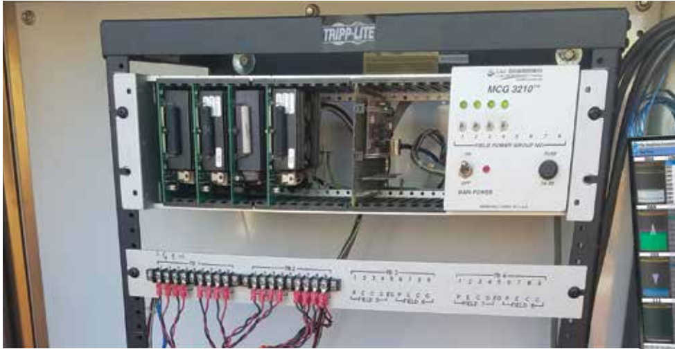
Photo of MCG 3210 Field Interface Card Rack.
