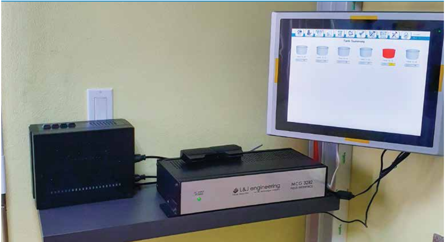
Photo of the High Level Alarm (HLA) System installed in the control room.
